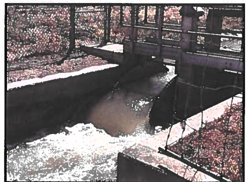
Irrigation district canal automated gate system—Hidalgo
