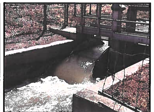
Irrigation district canal automated gate system—Hidalgo
